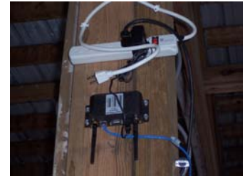
Figure 2. Cellular modem and power strip.
